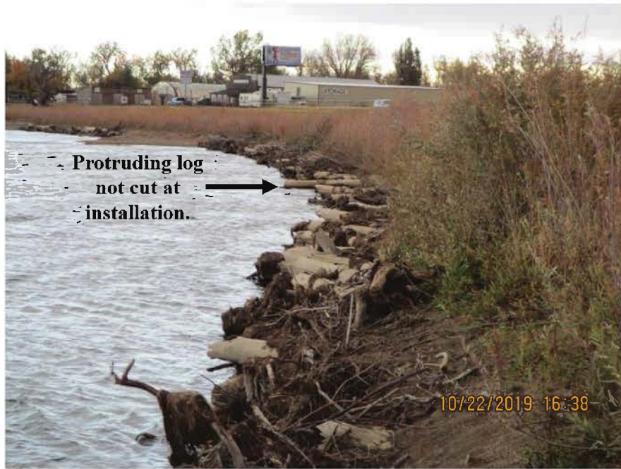
FIGURE A.5.1. Site 2 & 3 - Wyoming Blvd, standing near upstream end of toe wood 1, looking downstream.
