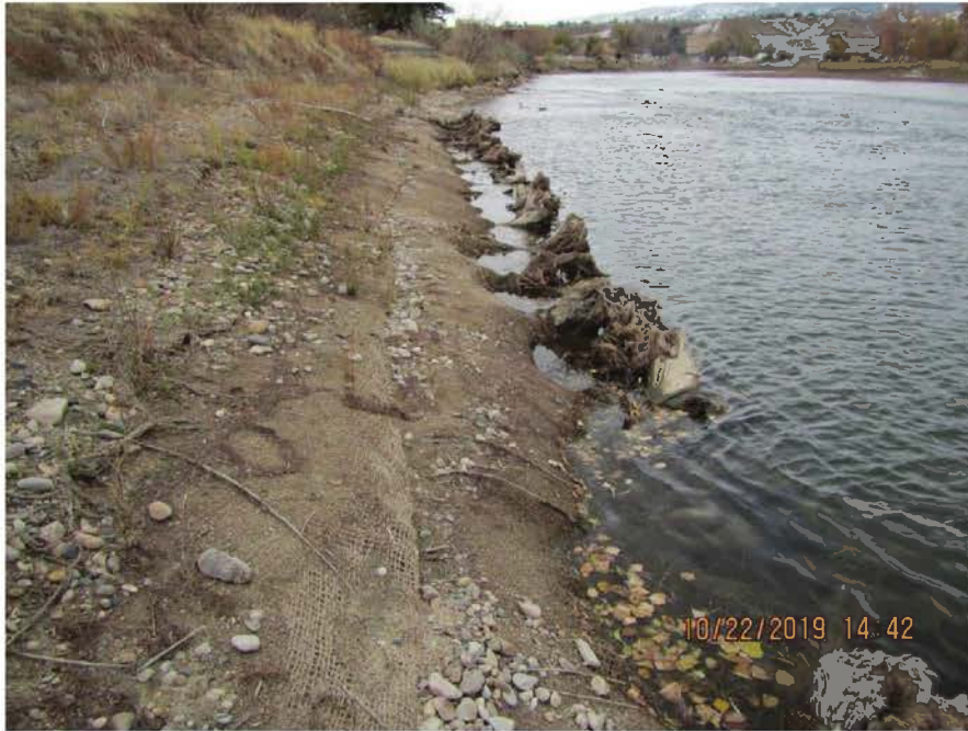
FIGURE A.5.7. Site 2 & 3 - Wyoming Blvd, standing at middle of toe wood 4, looking upstream at upper half of toe wood 4.
