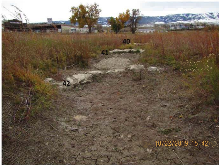
FIGURE A.5.23. Site 2 & 3 - Wyoming Blvd, at downstream set of wetland cross vanes, looking up at cross vanes 40,41, and 42.
