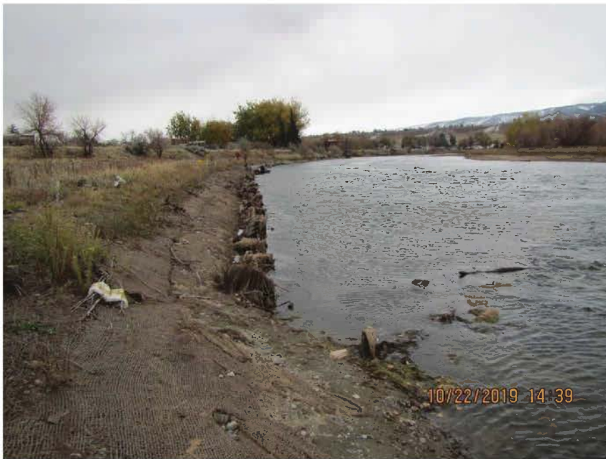
FIGURE A.5.8. Site 2 & 3 - Wyoming Blvd, standing downstream of toe wood 4, looking upstream at toe wood 4.
